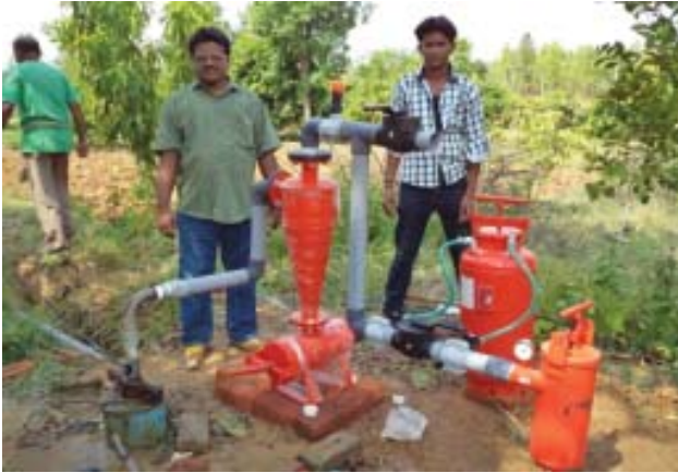
Drip irrigation in ITDA, Th. Rampur
