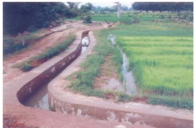
Const. of Canal system of Suakati Nalla in Tangarpada GP under Patna Block, Est. Cost- Rs.5.00 Lakhs, Year-2010-11, Scheme - SCA to TSP
