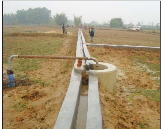
Construction of Field Channel of Dhobani L.I. Point taken up out of CCD Plan with an estimated cost Rs. 3.00 Lakhs during the year 2011-12. This provides water distribution system to the cultivated lands of LODHA PTGs of village Dhobani and near by villages
